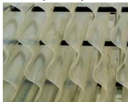
● Sludge thickening lamellas
