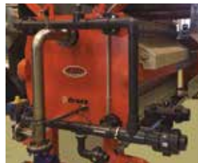
● Manifold in PVC
